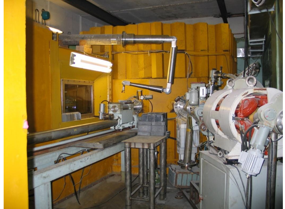
Isotope production facility
